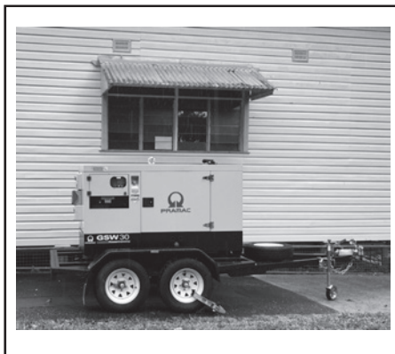
RUKI's trailer generator, donated by Tweed Shire Council, provided power at the community hub
