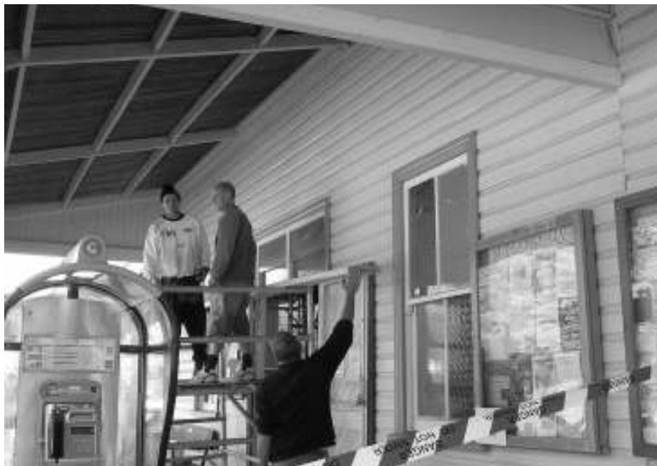
Hard at work on the essential repairs to the Hall. Photo by Jayne Parrott
